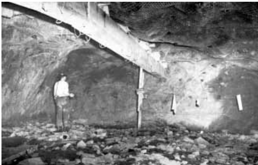
Figure 3. The large room where the tank will be installed in the Homestake Mine is shown about half-excavated, in the summer of 1965. From Sharp Bits , September 1965, published by the Homestake Mining Company.
