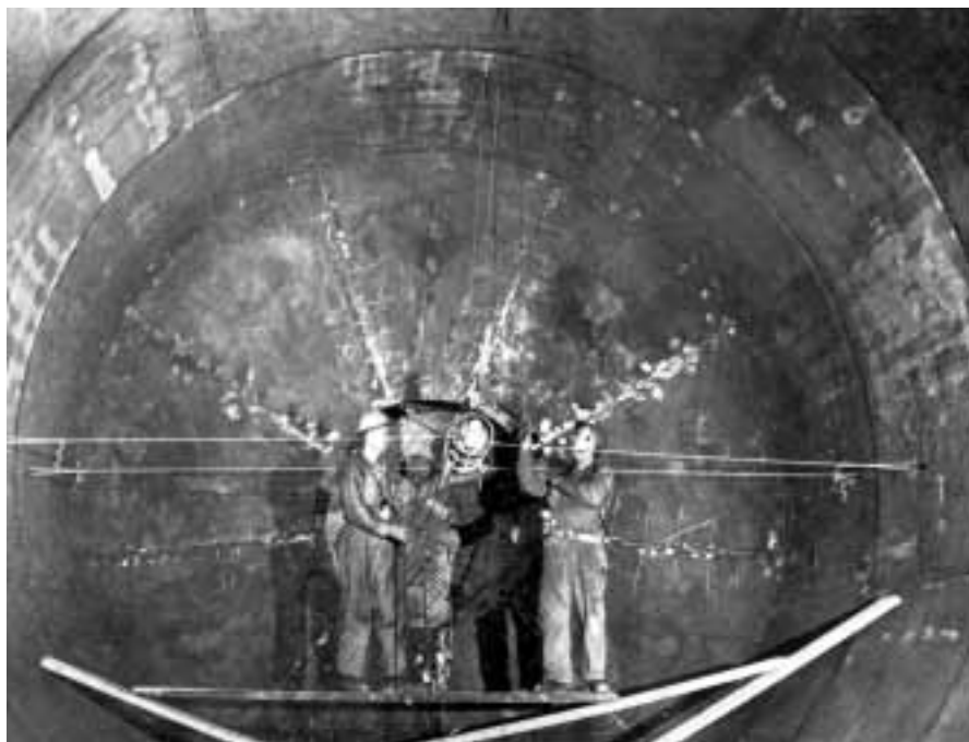
Figure 5. An X-ray source was placed at the axis of the tank and x-ray film was attached to the outside of the tank, in order to test all of the welds. From Sharp Bits , June 1966.
